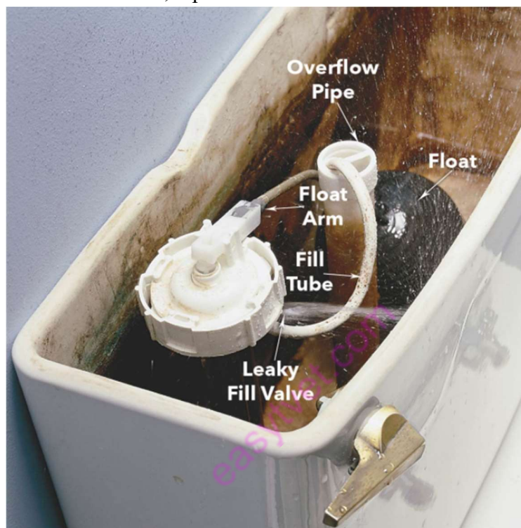
Check the fill valve
