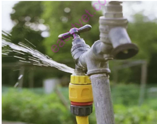
leaking hose bibb
